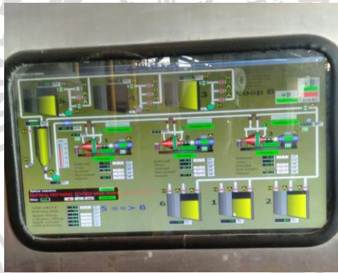
Gambar 2.7 Tampilan Monitoring Mesin Refiner.
