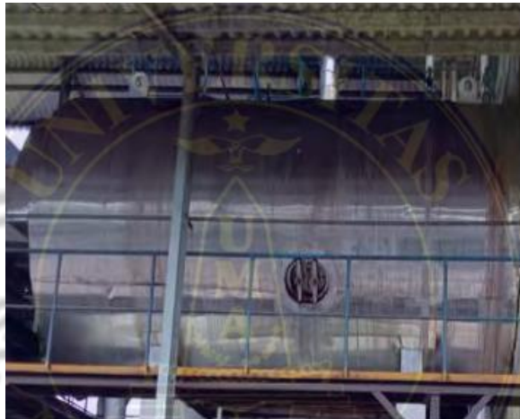
Gambar 2. 3 Steam Drum boiler Sumber (HASIBUAN J., 2023)
