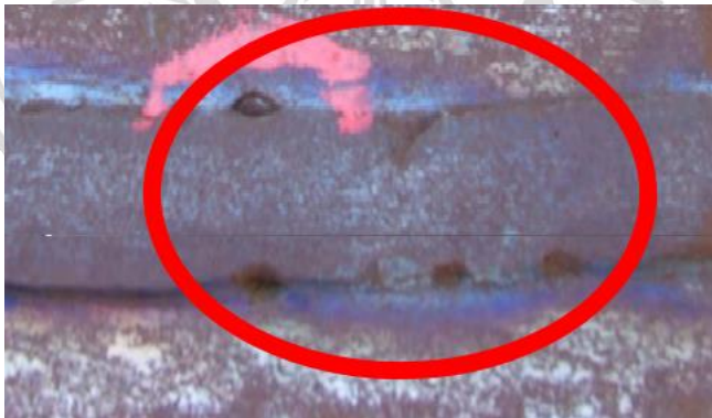
Gambar 4. 4 Defect Las Undercut
