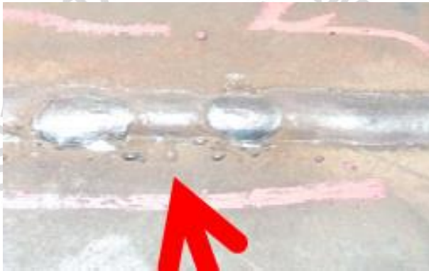
Gambar 4. 5 Defect Las Over Spatter
