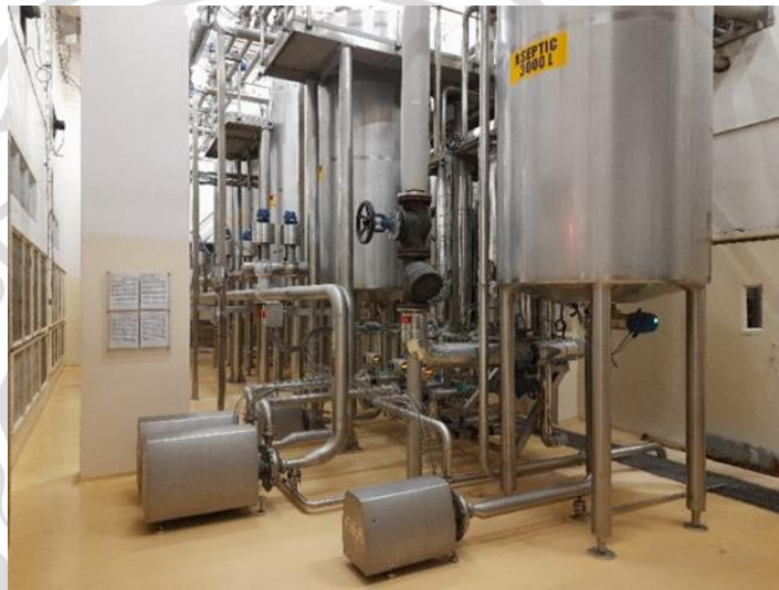
Gambar 1.5 Clean In Place (CIP) Plant
